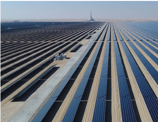
Source: Mohammed bin Rashid Al Maktoum Solar Park
